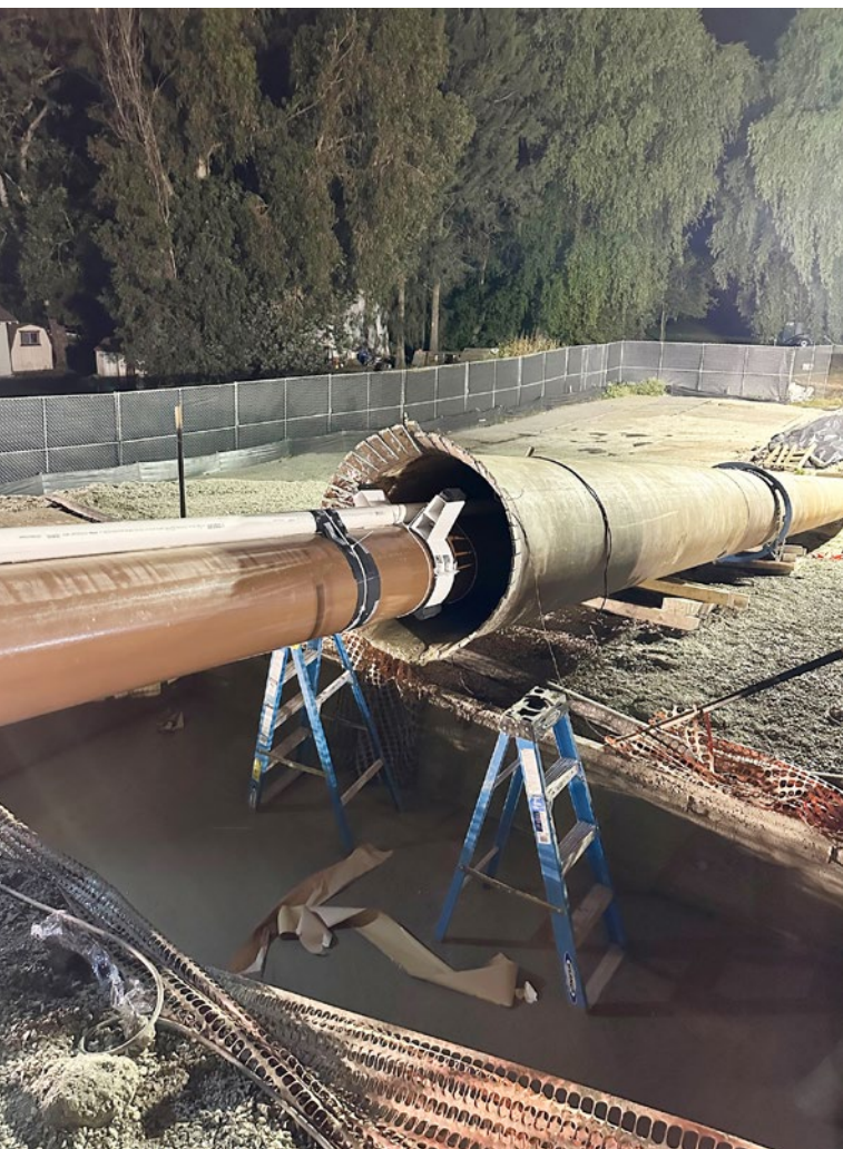
Figure 12. Casing spacers and PVC pipe for grouting the annular space being pulled into the eastern conductor casing
