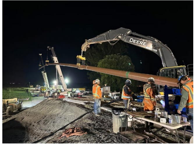
Figure 11. 16-inch gas pipeline nearing the end of pullback. Casing spacers were installed on the final 150 feet of the pipe after it came through the last roller cradle to centralize the product pipe inside the steel casing
