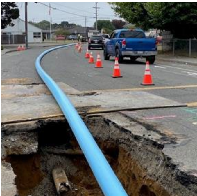
Figure 6. 8-inch FPVC being pulled in keeping one-way traffic flowing with minimal impact
