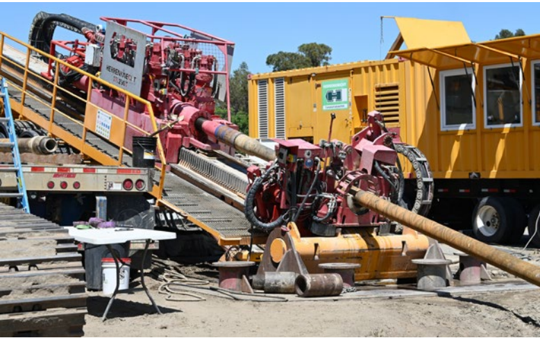
Figure 13. The primary HDD rig that was located in the western work area
