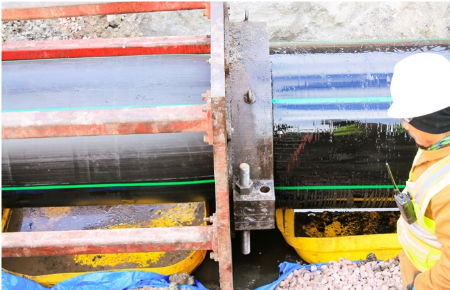
The new 36-inch HDPE pipe replaces the corroded ductile iron pipe in the Sioux Falls, SD sewer system (PHOTO CREDIT: MURPHY PIPELINE)
