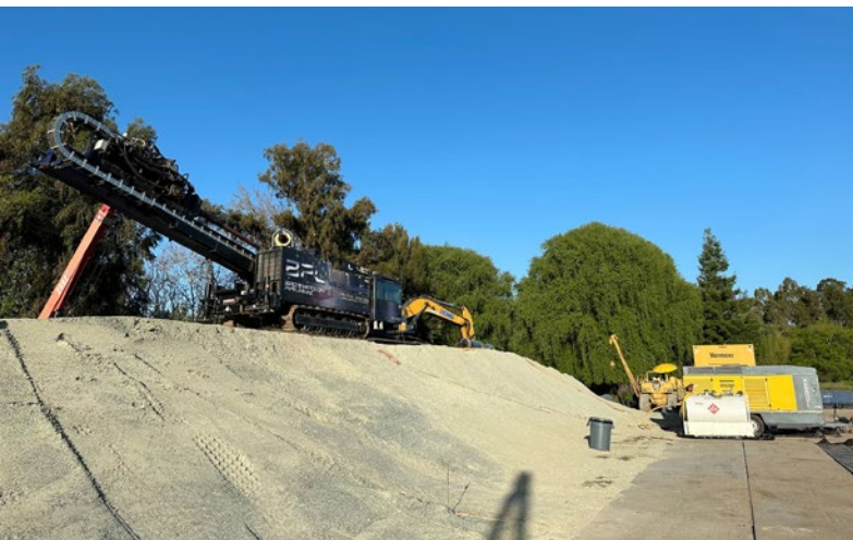
Figure 7. Brotherton's secondary HDD rig on top of the temporary work platform that was used to raise the eastern entry above the Sacramento River's mean high water elevation
