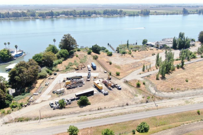
Figure 4. Aerial view of the western HDD work area looking across the Sacramento River project site
