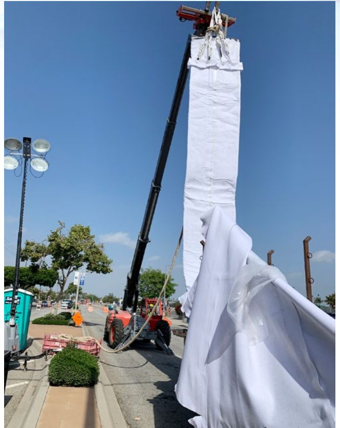
CIPP enables the LACSD to repair critical assets without utility conflicts or lengthy project duration
