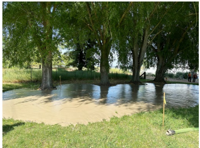
Figure 9. Drilling fluid from the hydrofracture near the end of the eastern conductor casing that occurred during pullback
