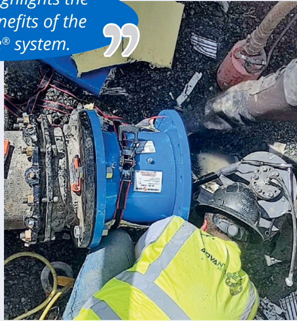
After connector assembly and pressure test, the rehabilitated pipeline could be reintegrated into the existing network. The installation had only taken two days
