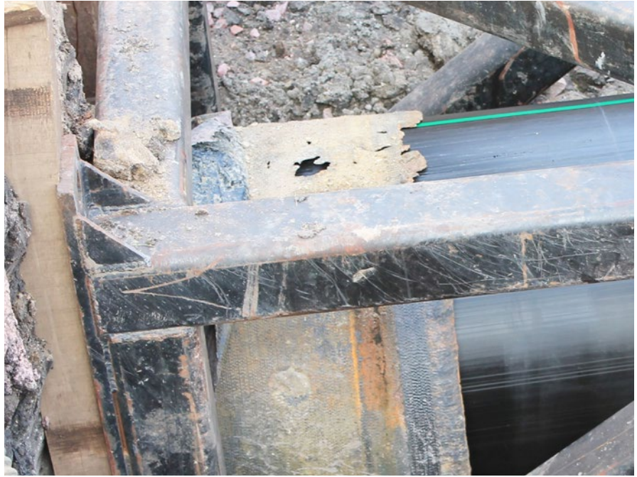
Replacing the Sioux Falls corroded ductile iron pipe that had been eaten away by sulfuric acid caused by sewage, the HDPE pipe is inserted into the destroyed pipe using the CompressionFit method from Murphy Pipeline (PHOTO CREDIT: MURPHY PIPELINE)
